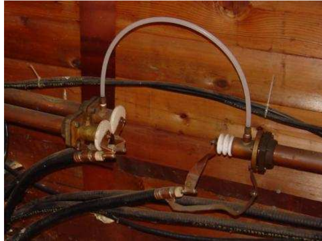
Figure 14.52: Flexible coaxial cables connected to rigid lines.
